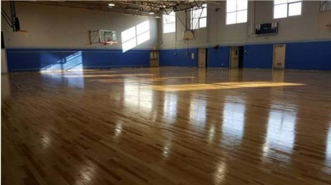
The new maple floor is down, has been sanded and has received a few clear coats.
